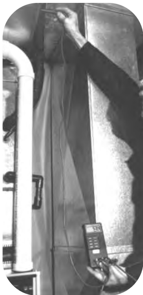
FIGURE 45 TEMPERATURE RISE MEASUREMENT
